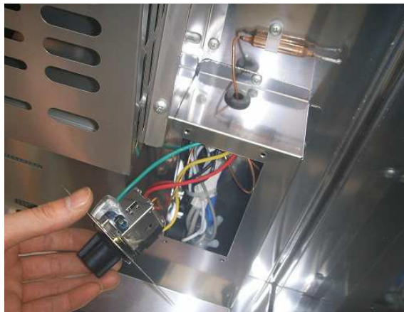
TEMPERATURE CONTROL & EVAPORATOR
